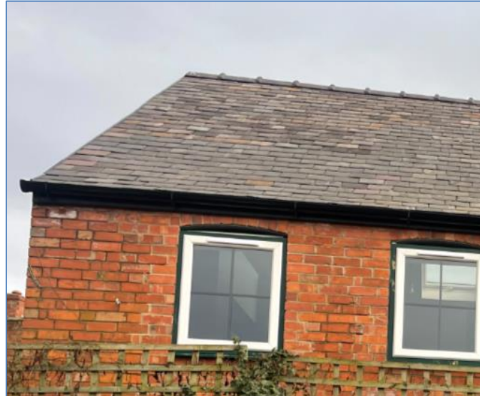
Site photo of (incorrect) windows originally installed.
