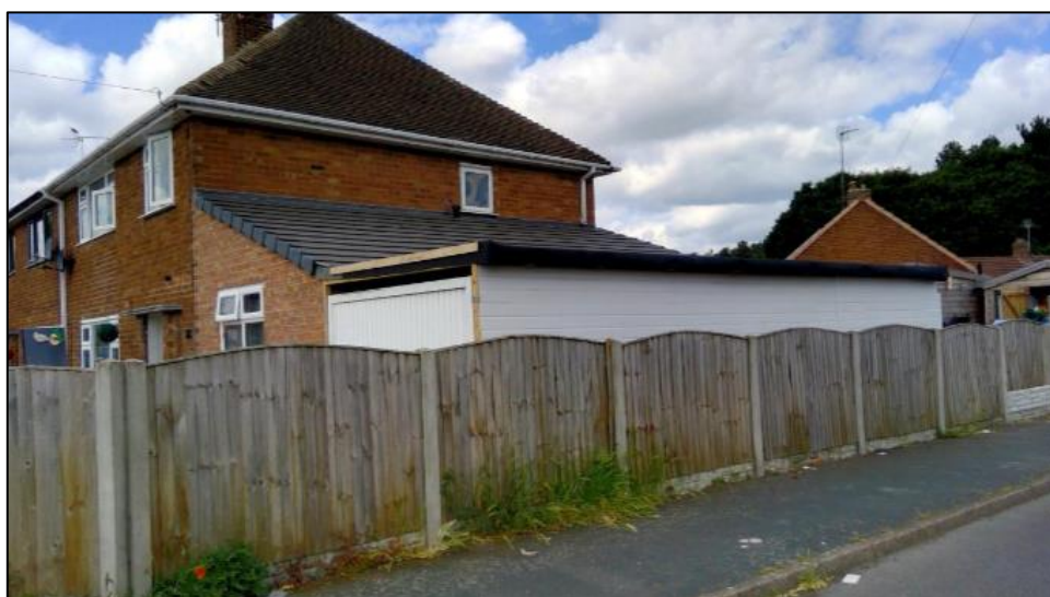
Site photo showing the unauthorised development.
